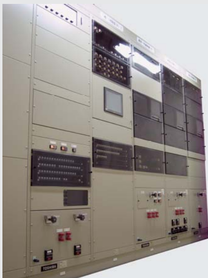
▲ 制御保護装置 Newly installed control and protection panels
